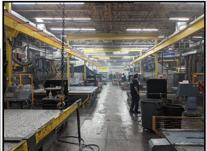
Mist-Free Shop Air after Micro Air Installation
