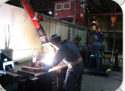
Source Capture Arms ducted to ceiling hung cartridge collector.
