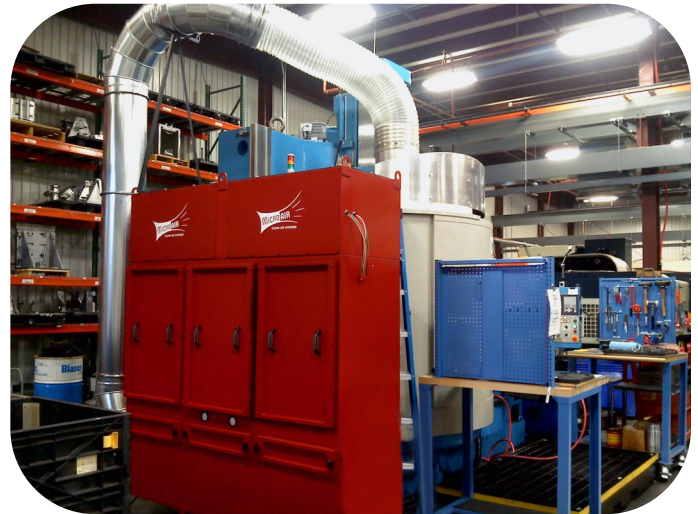
MM3600— Ducted to Machining Process
