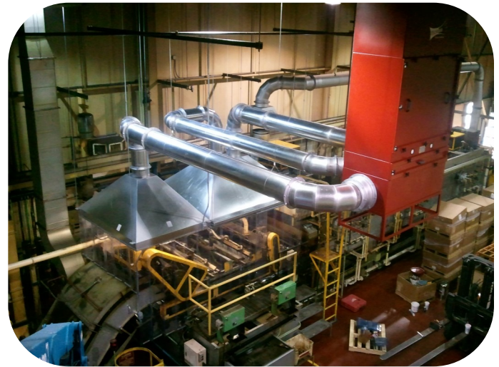
MM2400—Ceiling Hung Ducted to Hoods over Machining Process
