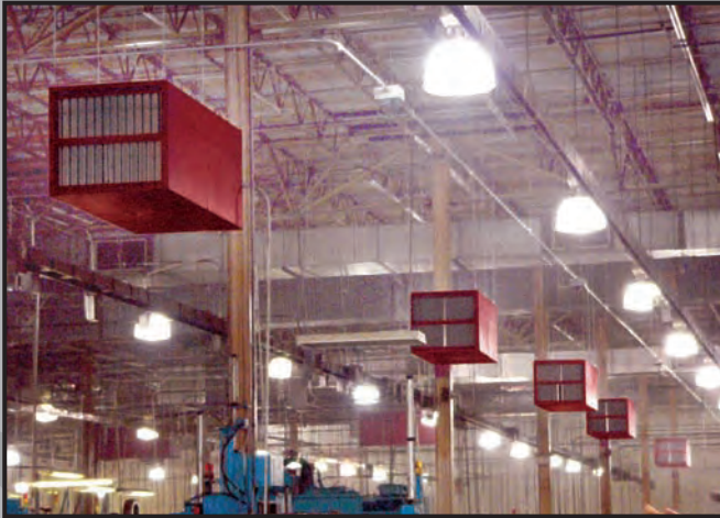
Horizontal 6000 cfm Mist collectors mounted in race-track Configuration for ambient capture of mist.
